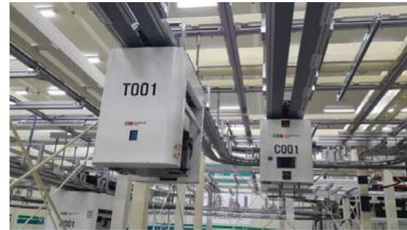
Overhead Hoisting Transport
